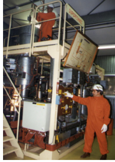
FIG. 2. Trainees working on the filling of a sodium loop (the Sodium School).
