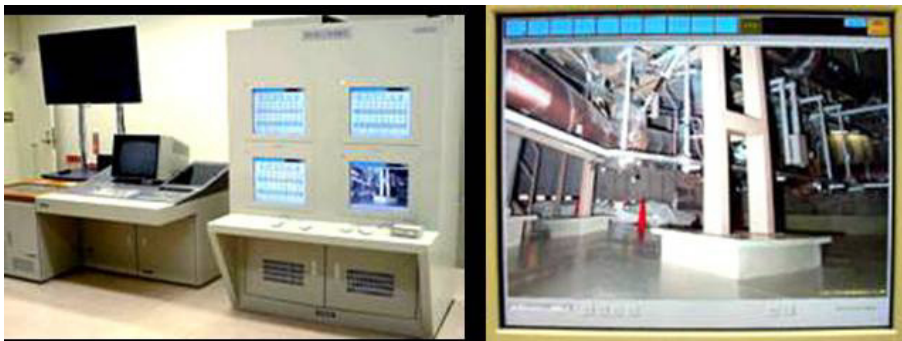
FIG. 5. Synthetic sodium leak monitoring system.
